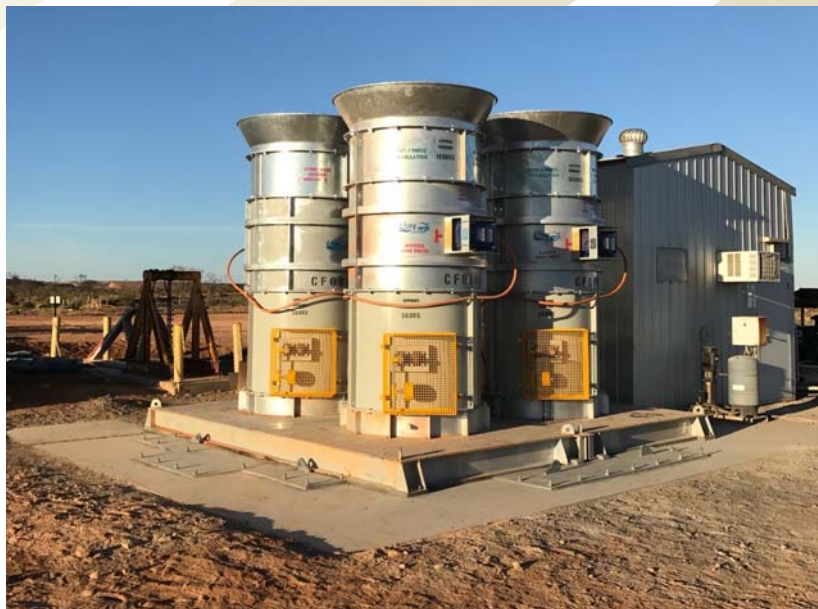
Figure 1: primary fan bank at the ventilation shaft collar fully installed and running
